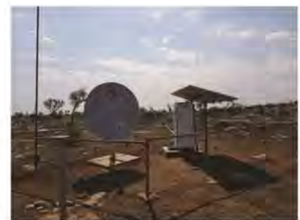
Image courtesy of Geoscience Australia. Image outlines an indicative setup of a seismic monitoring station.
